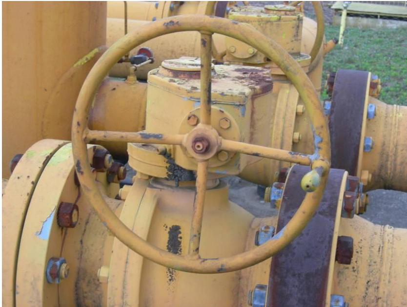
Figure 3 Distribution network valve
